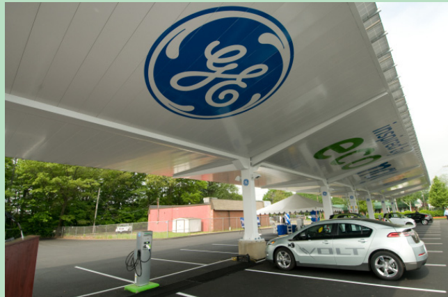
Figure 9: General Electric's Solar Carport, installed in Plainview, Connecticut (Source: GE, courtesy of C|Net).
