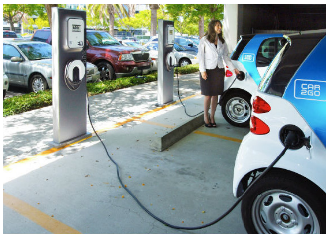
Figure 8: San Diego's first EVSE, in a real estate company's parking garage. (Source: www.hybridcars.com ).
