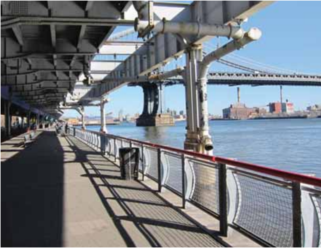
Existing esplanade along South Street underneath the FDR Drive, with downspouts emptying into the East River
