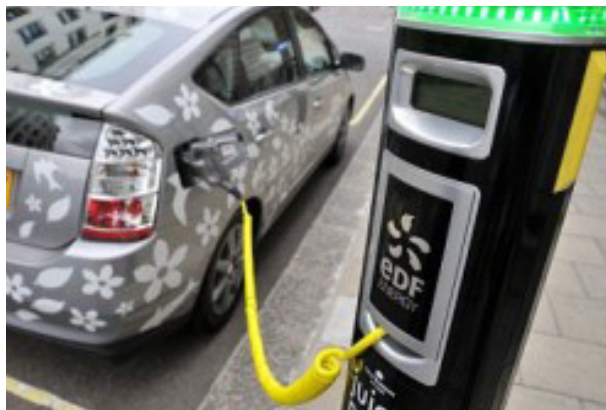
IMAGE 5. LONDON, UK CORD MANAGEMENT TECHNOLOGY AND EVSE PLACEMENT IS ESPECIALLY IMPORTANT FOR ON-STREET PARKING SO AS TO NOT CREATE TRIPPING HAZARDS. EVSE SHOULD NOT BE PLACED IN A LOCATION THAT WOULD CROSS SIDEWALKS OR PEDESTRIAN PATHS. RETRACTION DEVICES OR A PLACE TO HANG PERMANENT CORDS AND CONNECTORS SUFFICIENTLY ABOVE THE GROUND SHOULD BE PRESENT ON ALL EVSE.
