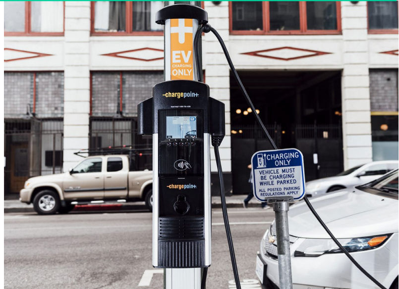
Figure 34: ChargePoint dual-port installation in Los Angeles.
